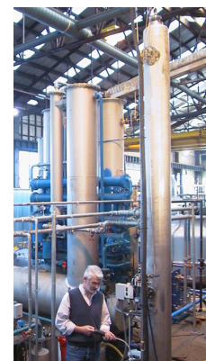
High pressure purifier
