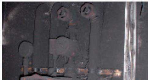
Fire damage before ...
