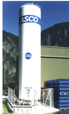
Vertical CO 2 storage tank
